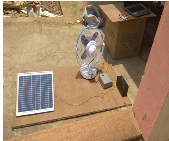
Fig 7: Connecting DC load with Battery
